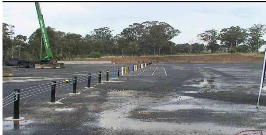
Wire Rope Barrier
